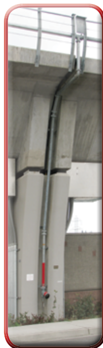
Elevated light railway protected by dry standpipe system with Storz connections. Knox® StorzGuard® protects coupling FDC from tampering
