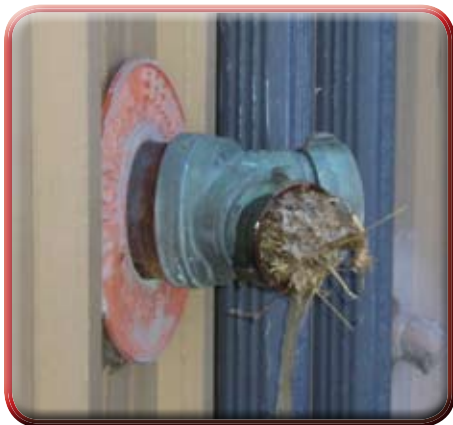
Accumulated debris will eventually require a backflush to keep FDCs serviceable. Photo courtesy of Moline, IL Fire Department
