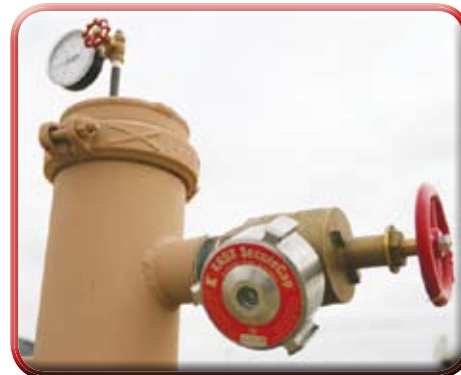
Knox SecureCap™ protecting a parking garage standpipe connection.
