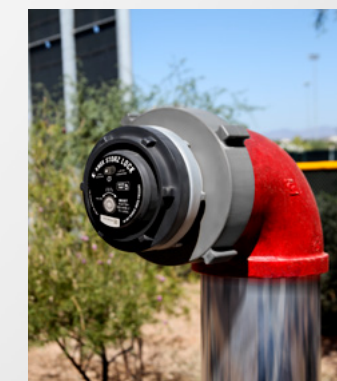
Knox Storz Lock secured onto a large FDC
